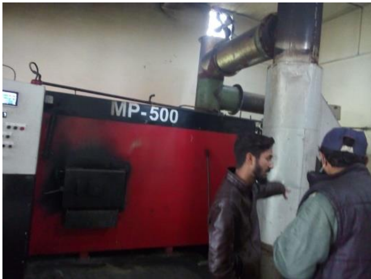
Waste incineration plant was installed in DHQ Hospital Jhelum (Para 4.5.3)
